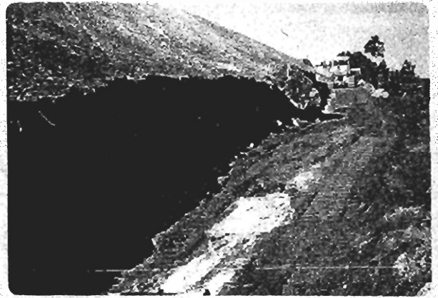
2. Berm Cut by Bulldozer, Note Grey Sand of Original Underdrain
